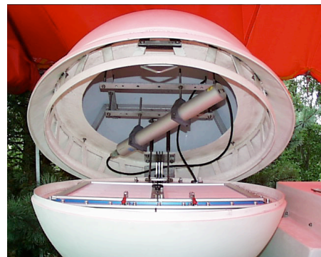
GM-probe installed to monitor particle filter radiation level
